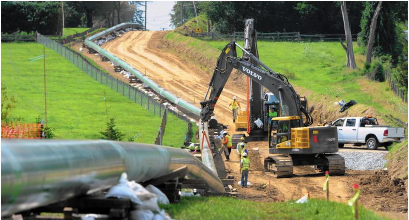
Crews worked on a section of a new four-mile Baltimore Gas and Electric natural gas pipeline along Route 136 in Churchville in 2014. (Matt Button/Aegis). (MATT BUTTON | AEGIS STAFF, Baltimore Sun Media Group)
