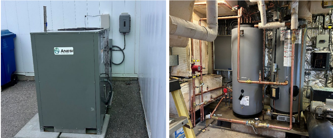
Figure 10. Installed GHP and Pre-Heat Tank at Site X
